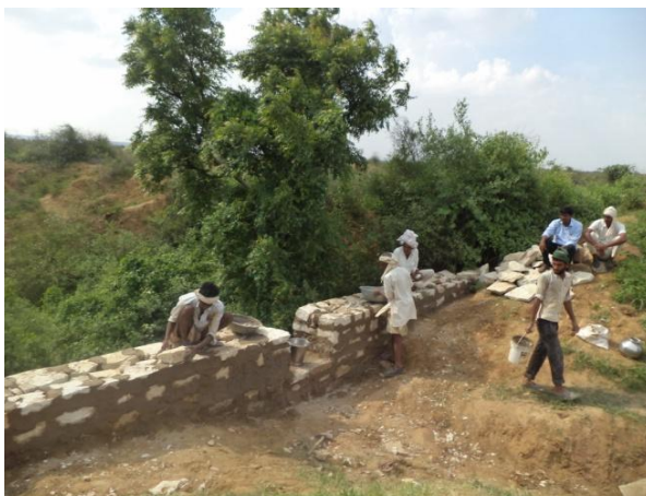
Jal NikashNaali (Water Drain System)
